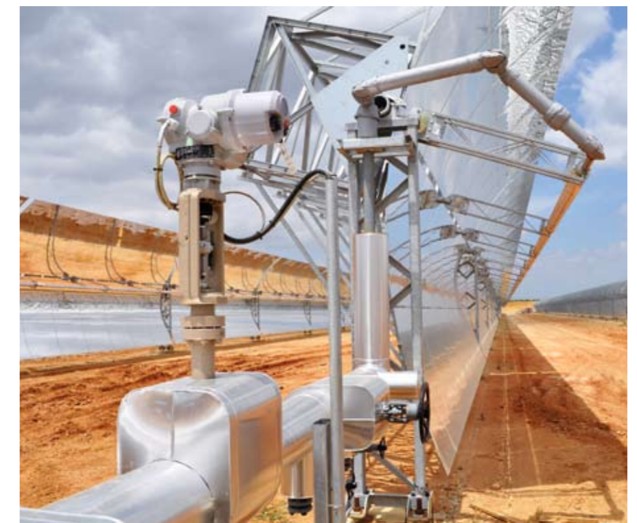
The trough collectors heat the transfer oil up to reach temperatures of 400 °C. 168 Type 3251 Control Valves in NPS 3, Class 600 with bellows and electric actuators ensure optimum flow.
