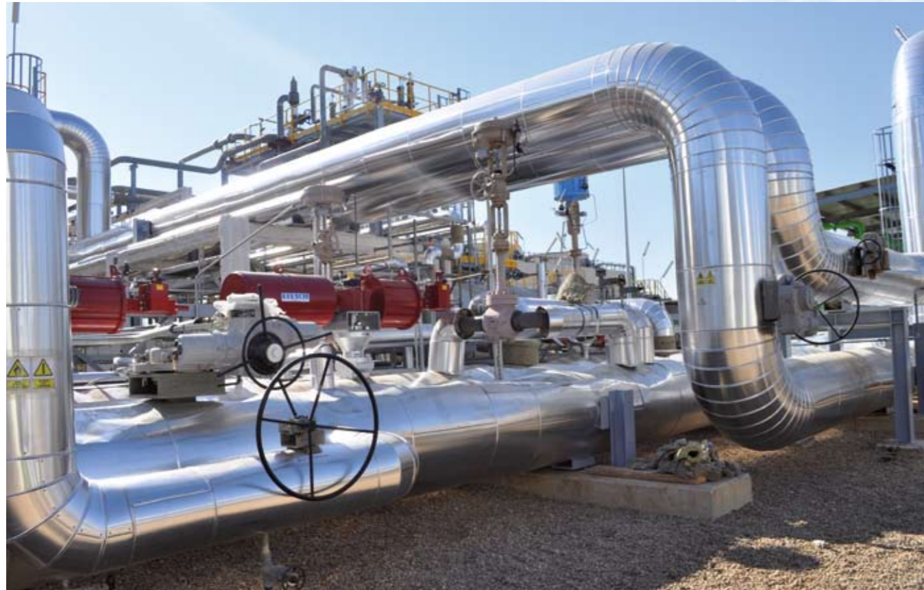
In the SAMCASOL plant, the flow rate and temperature of the heat transfer oil, which is routed through the entire solar field to the power plant, are regulated by a LEUSCH LTR 43 Butterfly Valve and a SAMSON Type 3241 Valve in split-range operation.
